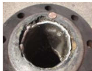
Severe Flange Corrosion
